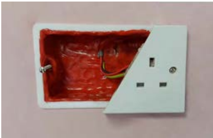
Actual installation of a Quelfire Putty Pad Installed Flush with the Front Face of the Plastic Socket Box
