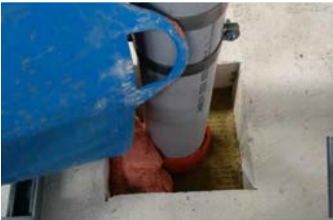
QWW CE Marked Intuwrap installed in an oversized hole sealed with QF2 Fire Protection Compound in concrete slab
