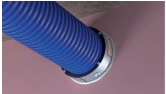
QRS CE Marked Intumescent Fire Sleeve (circular) installed around semi-rigid duct in plasterboard partition
