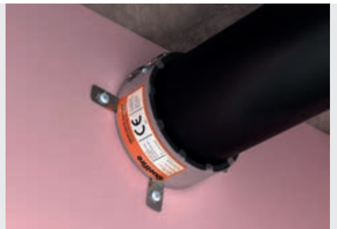
QWR CE Marked Fire Collar installed on plasterboard wall
