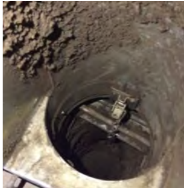
These pictures show extreme build up of debris found by our team in ductwork. The 'fresh air' in these buildings passes through this filth!
